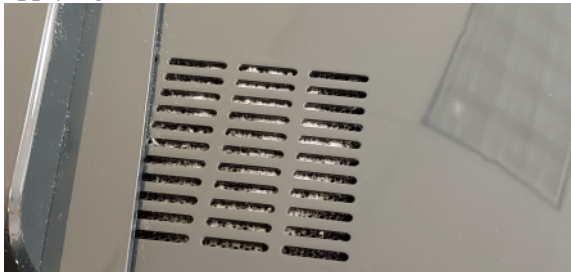
Clogged Cooling Vent
